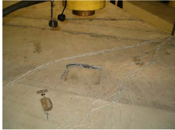
Figure 57 – Panel Punching Failure
