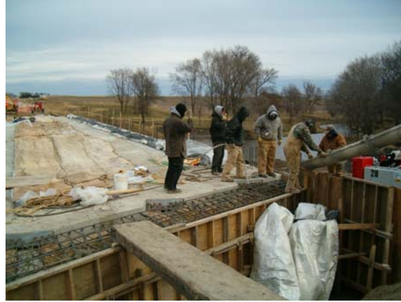
Figure 49 – CIP End Diaphragm
