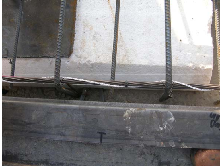
Figure 67 - Corrosion sensor installed on production box beam
