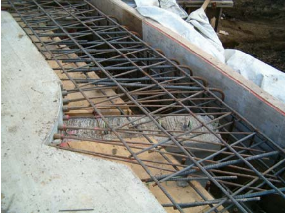
Figure 48 – CIP End Diaphragm
