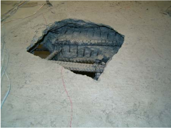
Figure 58 – Panel Punching Failure
