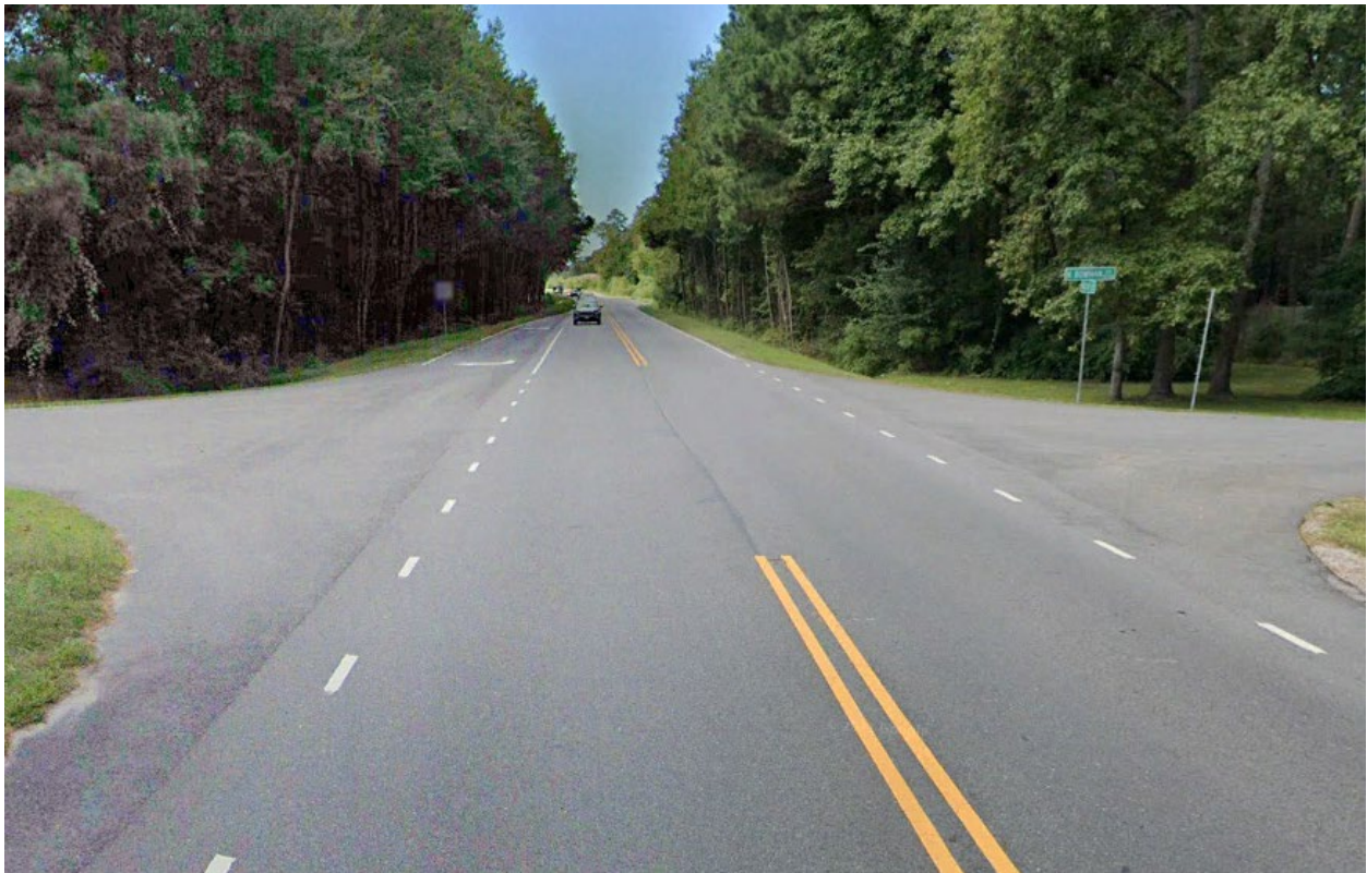
Photo 19. Edge line extension through the intersection and no passing zone markings on the approaches.
