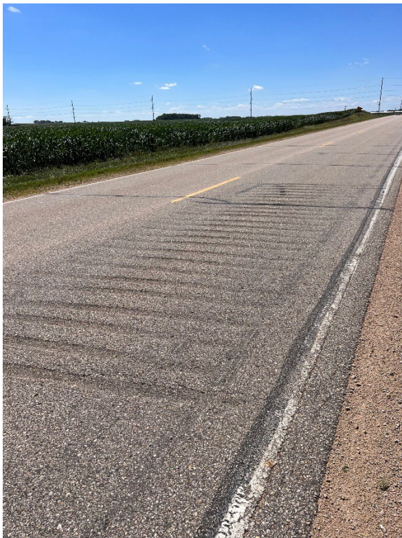
Photo 11. Tire path wear in rumble strip.
