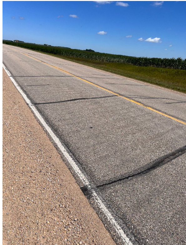
Photo 12. Tire path wear in rumble strip.
